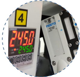
Festo pneumatics and OMRON temperature controllers
